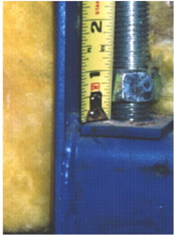
Figure 4. Five Stories – Ave. shrinkage 5/16" per floor.
